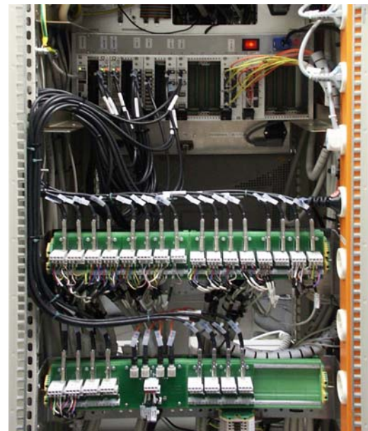
Fig. 2. Interlock Crate with distribution panels
